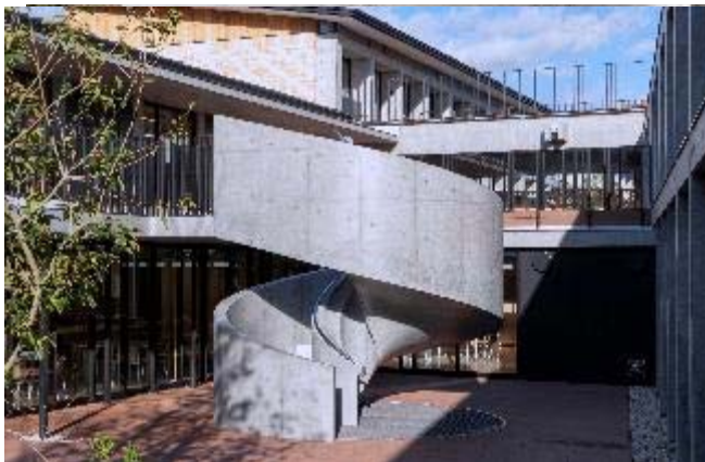
Air intake under spiral staircase
